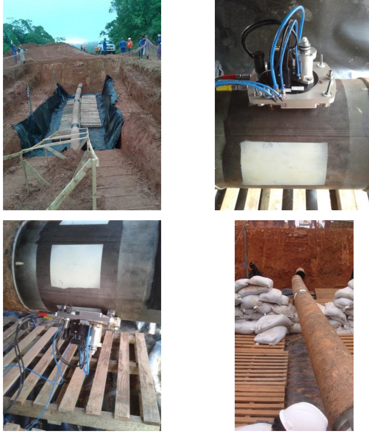
Fig 6. Application example (upper left), optical device (center), pipeline after cutting (bottom right).
